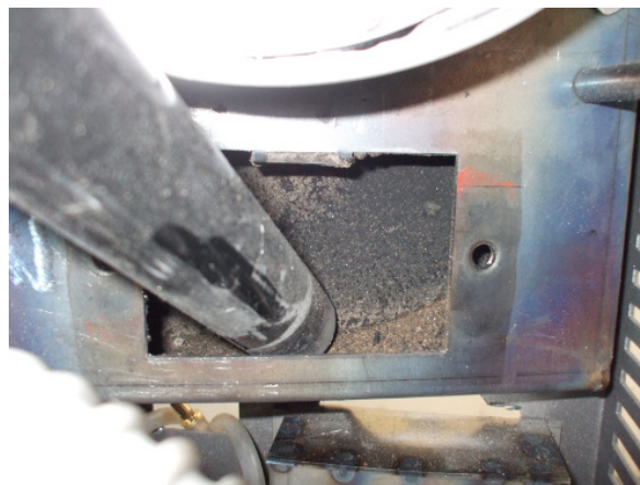
Fig. 47 - Fume chamber cleaning
